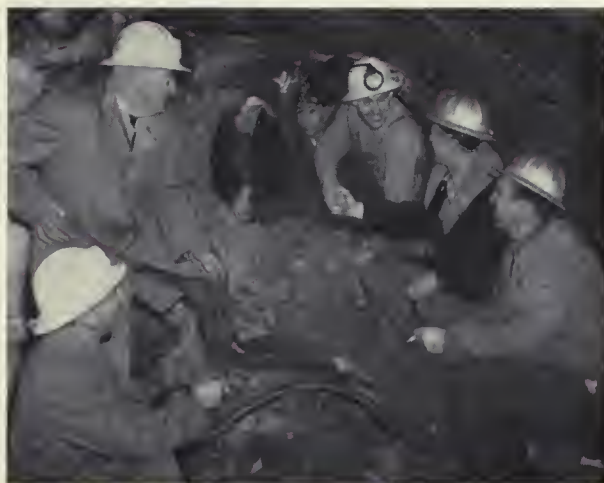
FROM EAST AND WEST—They “holed through” Pole Hill Tunnel on March 15, 1951. After the final blast the usual handshakes from those on the two ends of the tunnel were exchanged. D. E. Cortee, hard-rock miner who helped set off the final blast, receives his handshake from J. H. Knights, district manager, Bureau of Reclamation. Looking on are (at extreme left) Robert Barkley, engineer, Northern Colorado Water Conservancy District, Greeley, Colo., J. M. Dille, secretary-manager, northern Colorado Water Conservancy District, Fort Morgan, Colo., Ren Read, assistant district manager, Bureau of Reclamation, and an unidentified miner. At the extreme right is K. W. Dickey, Bureau of Reclamation field engineer. The Wunderlich Company was the contractor for drilling the 5.6 mile tunnel, part of the Colorado-Big Thompson project, in record time. They started work in September 1949, and holed through in 75 percent of the time anticipated for this part of the job. Photo by N. T. Novitt, Region 7 photographer.
